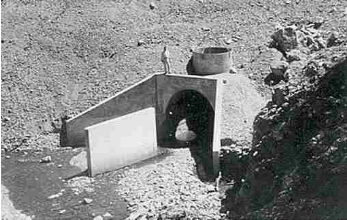
Figure 5.32. Combined installation of concrete debris fin and metal pipe debris riser with single corrugated metal pipe culvert (looking downstream).
