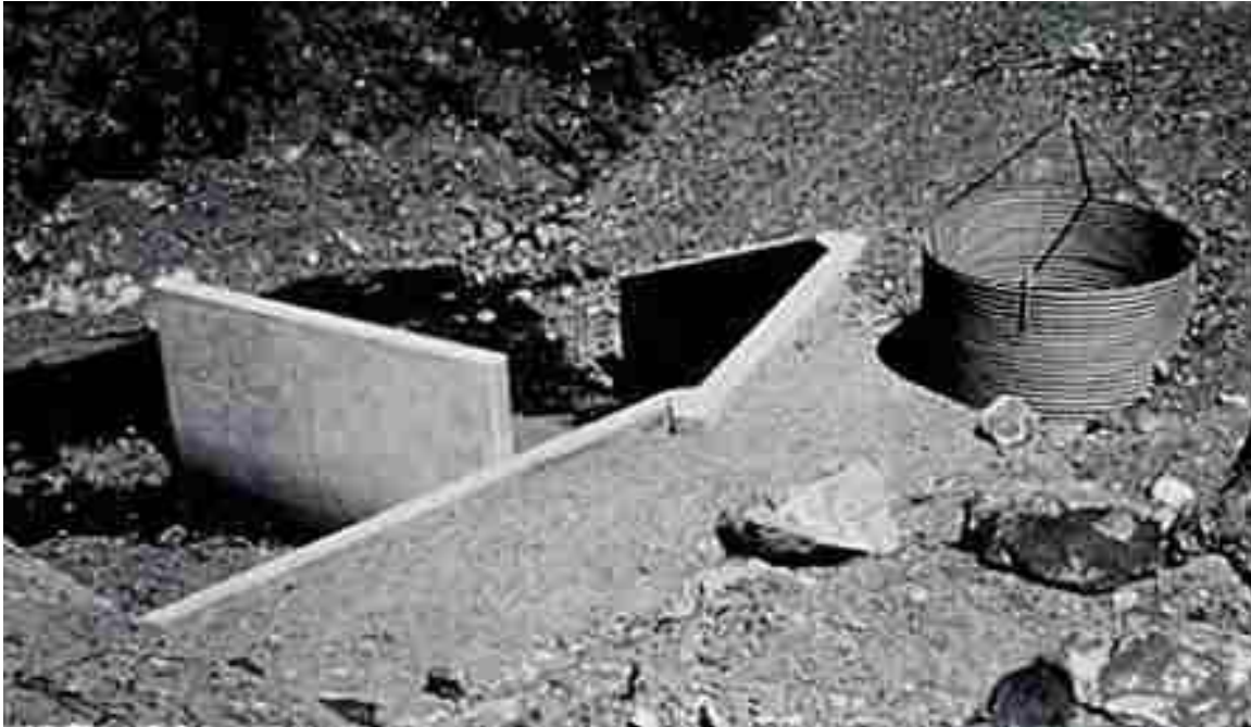
Figure 5.34. Debris fin and metal pipe debris riser in conjunction with single barrel culvert.
