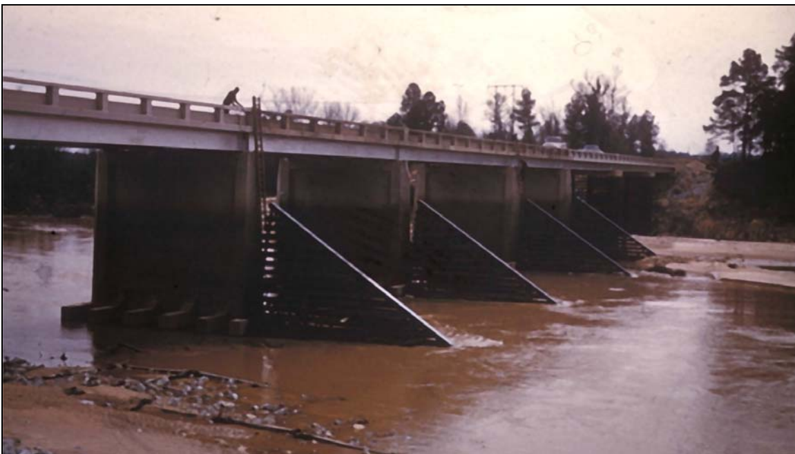
Figure 5.35. Timber debris fins with sloping leading edge.
