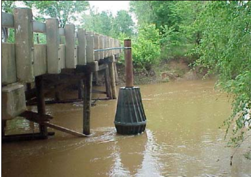
Figure 5.46. Close up of a debris sweeper installed on the South Fork Obion River in Tennessee.
