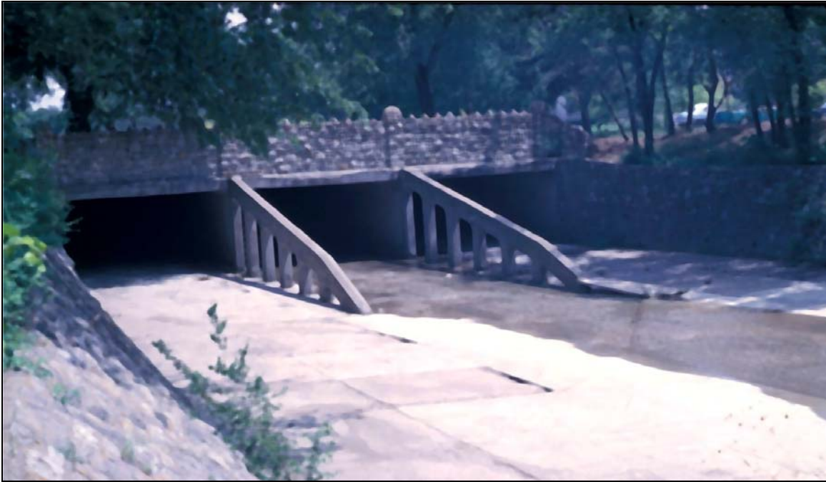
Figure 5.29. Concrete debris fins with sloping leading edge as extension of culvert walls.
