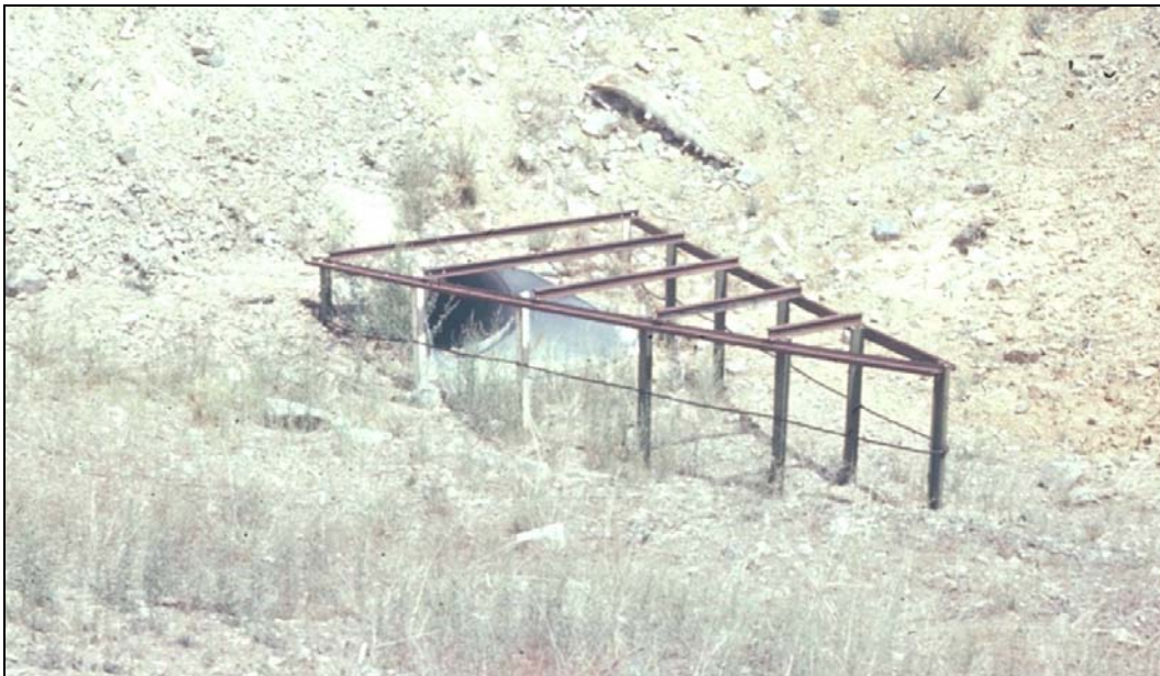
Figure 5.3. Steel rail and cable debris deflector. In boulder areas, cable is more desirable for its flexibility than a rigid rail (looking towards entrance).
