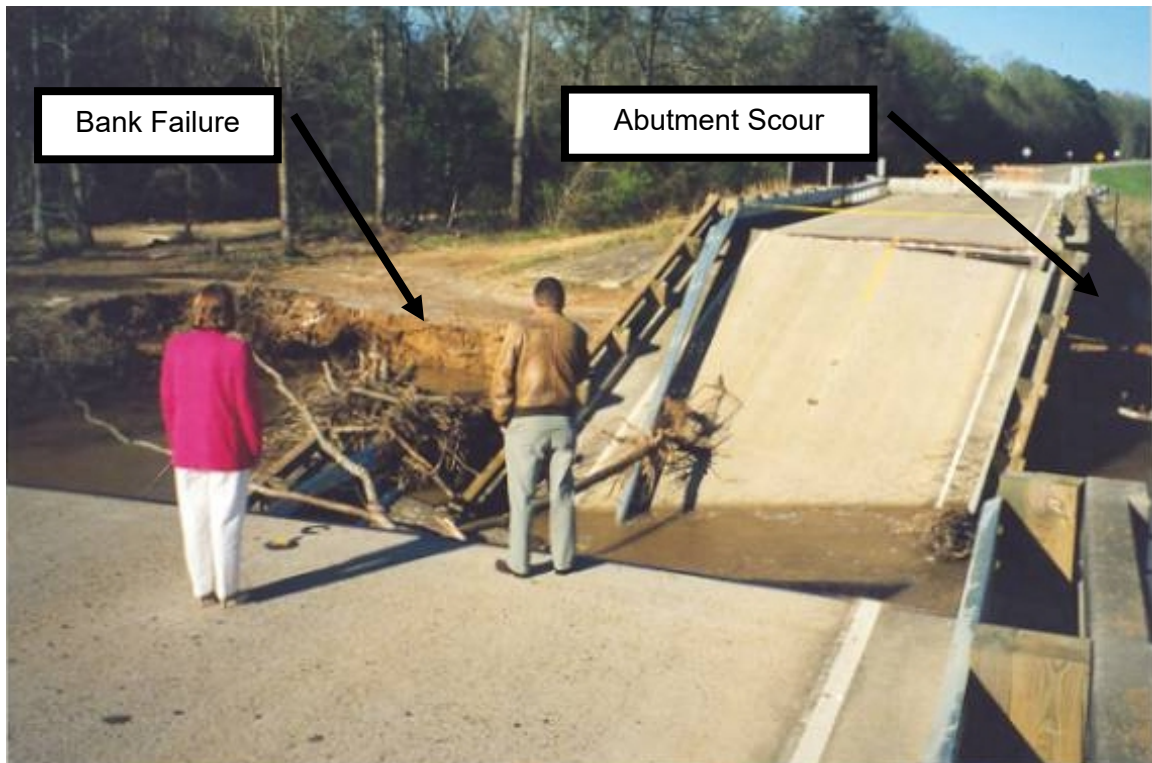
Figure 2.7. Debris induced bridge and bank failure structure. (Louisiana)
