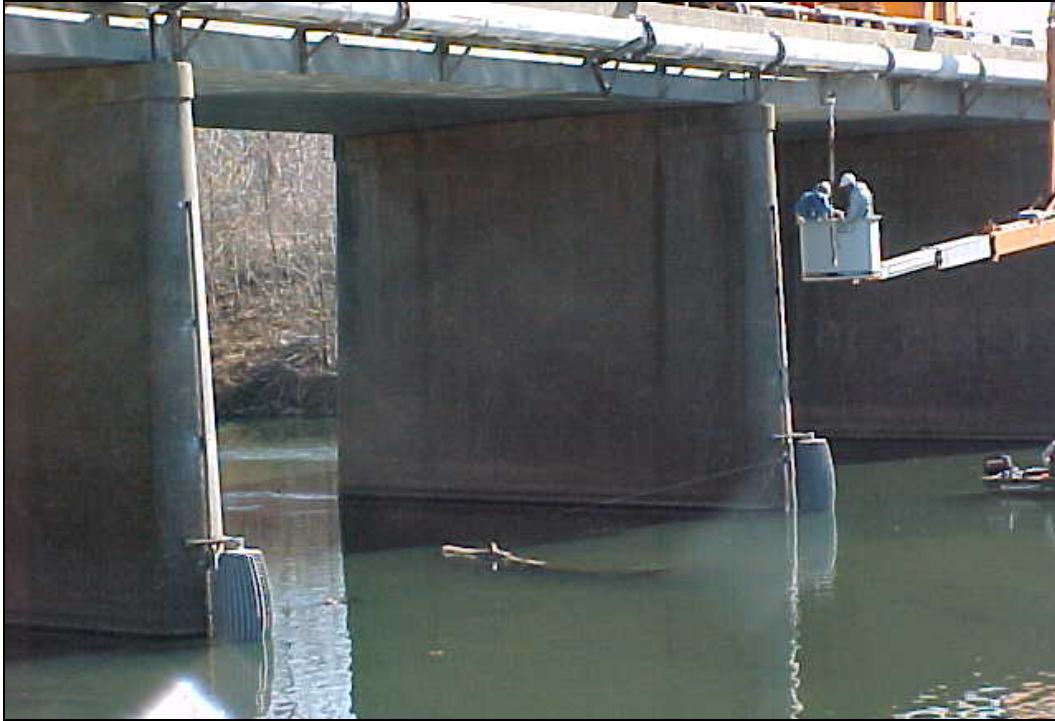
Figure 5.44. Debris sweeper being installed on a bridge over Staunton River in Altavista, Virginia.
