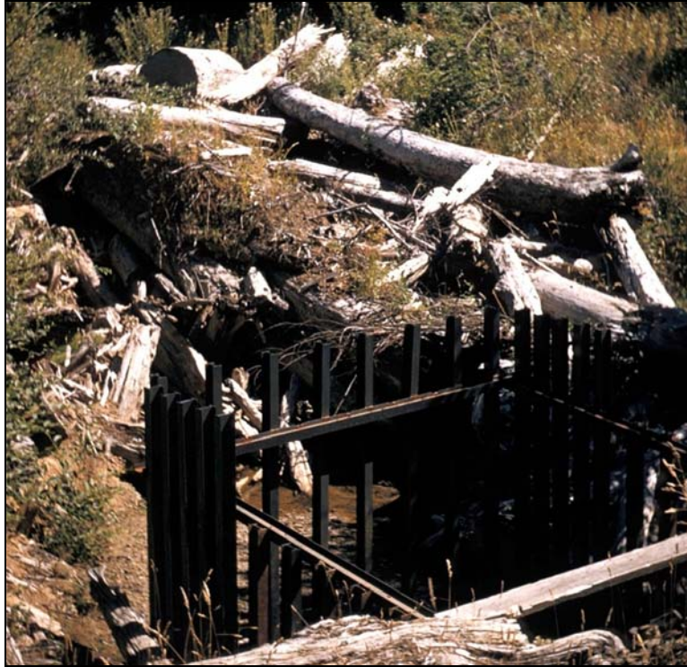
Figure 5.19. Steel rail debris rack. Note amount of debris accumulation in upstream channel.
