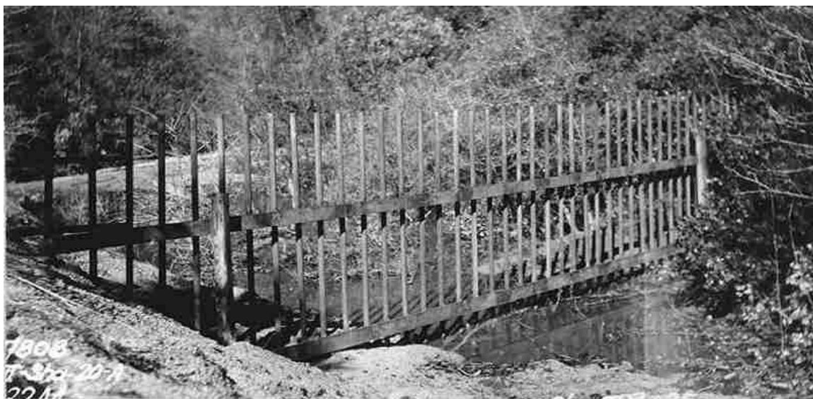
Figure 5.11. Post and rail debris rack, in place for 35 years, for light to medium floating debris installed 100 ft upstream of culvert.
