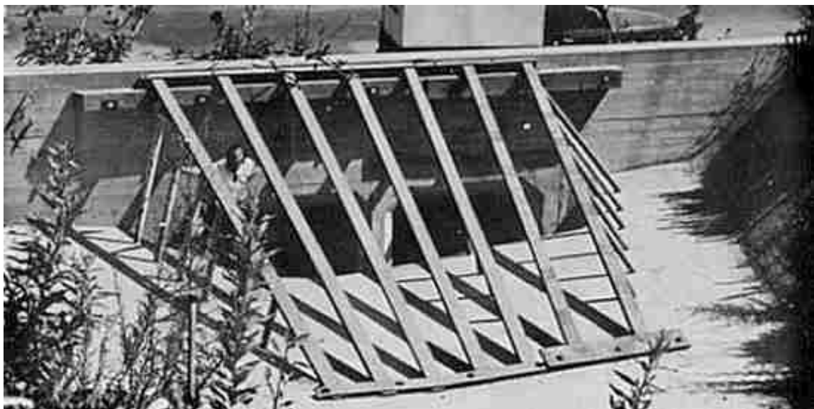
Figure 5.21. Steel grill debris rack with provision for cleanout afforded by concrete paved area in foreground.
