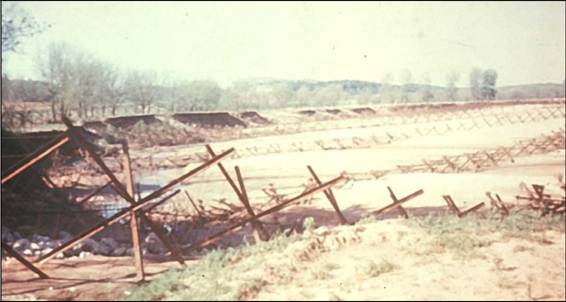
Figure 5.42. Kellner jacks used for redirecting the flow patterns.
