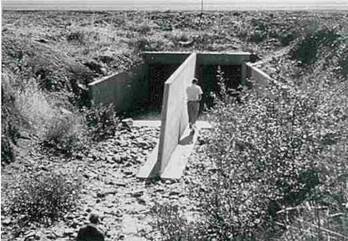
Figure 5.31. Concrete debris fin with rounded vertical leading edge as extension of culvert center wall.
