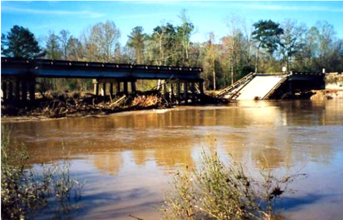
Figure 2.3. Span blockage accumulation bridge failure. (Louisiana)
