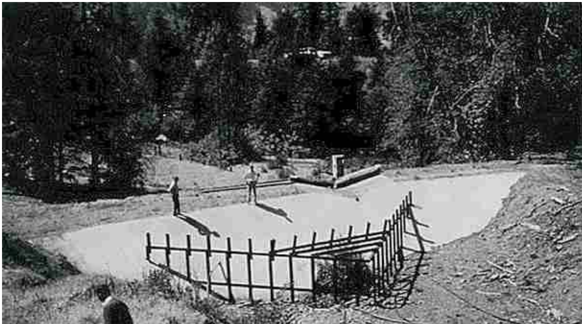
Figure 5.40. Debris dam and basin along with steel debris rack over culvert entrance in foreground. A metal pipe riser is visible over the spillway.
