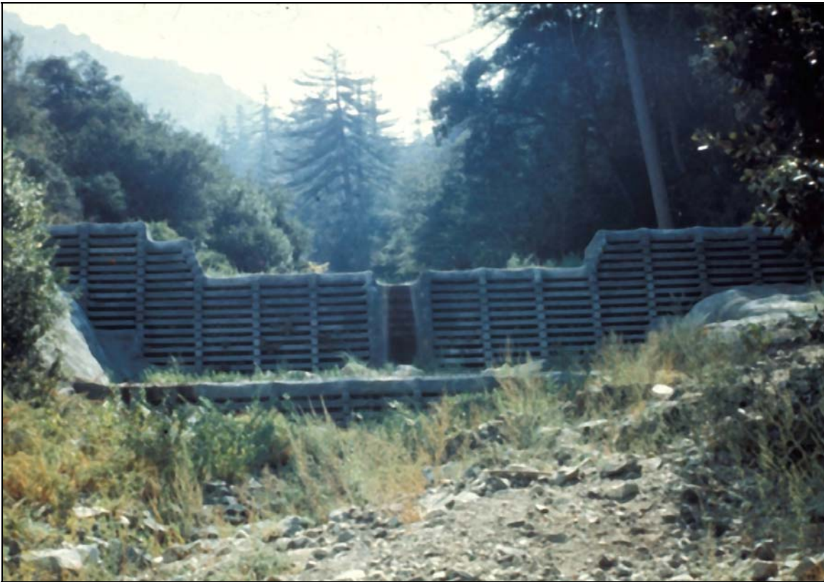
Figure 5.39. Debris dam of precast concrete sections fabricated to enable placement in interlocking fashion.
